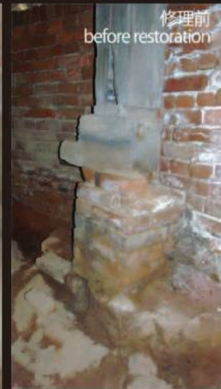
修理前 before restoration 焦げ跡が残る Burnt column end
